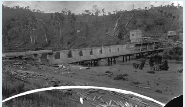
Figure 1: Mount Crosby Weir Bridge under construction in 1926. Source: State Library of Queensland.
