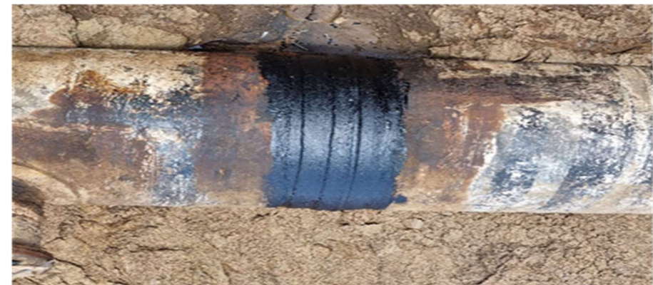
Figure 5: Rising main where the pipeline had slipped out of socket joint.
