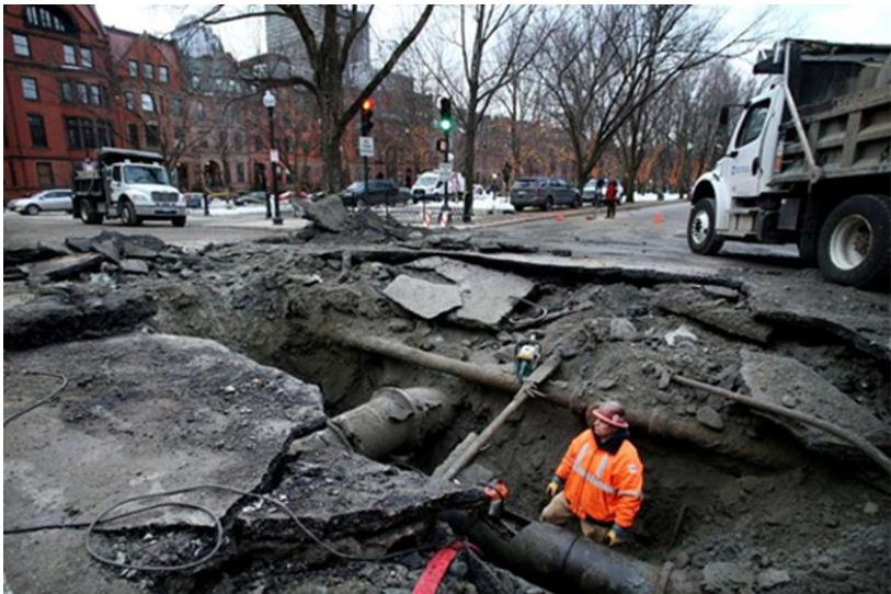
Figure 3 – An example of the damage caused following the break of a relatively small Trunk Water Main demonstrates its potential to render other community infrastructure unusable until repairs are completed.
